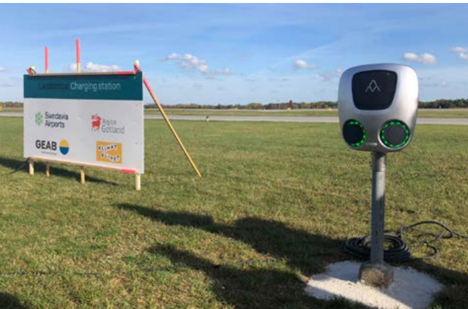
Charging post for electric aircraft at Visby Airport.
